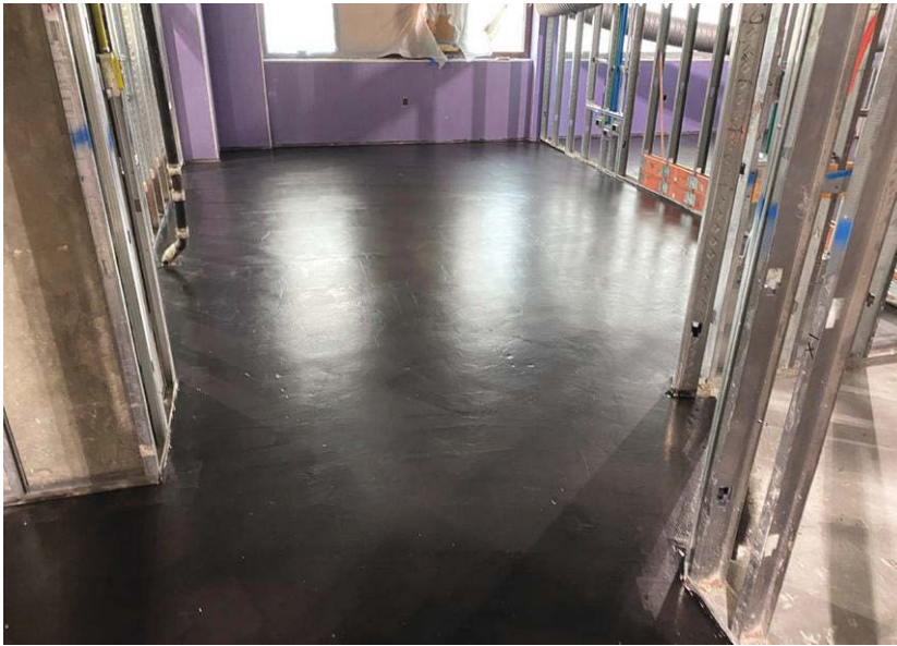
Left: The original flooring at Grady Memorial Hospital dates back to 1892 and renovations and additions over time created a variety of issues that needed to be addressed. As a first step, Ardex K 13 self-leveling underlayment was used to level and smooth the substrate to create a surface that would handle any type of resilient flooring.
